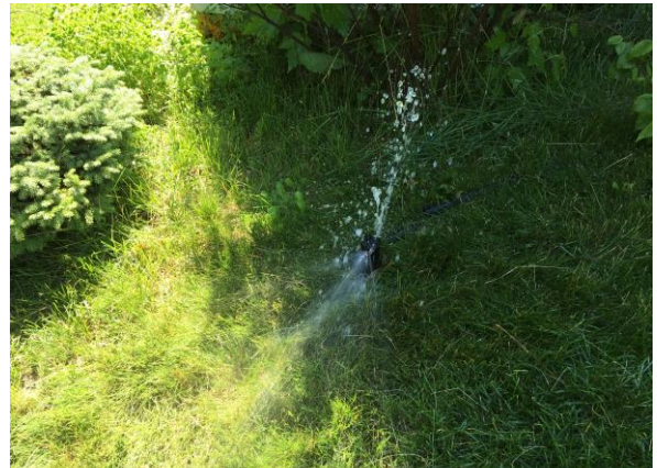
REPLACE BROKEN AND LEAKY SPRINKLERS
